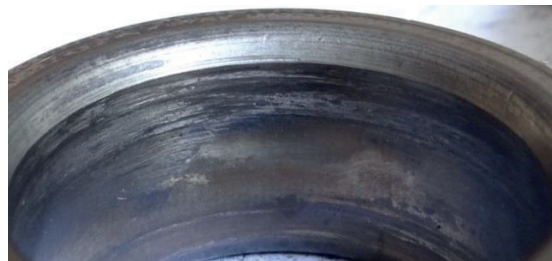
Smearing, polished surface of outer ring, fretting corrosion on inner ring bore
