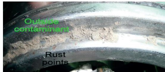
Corrosion. Contaminant deposit.
